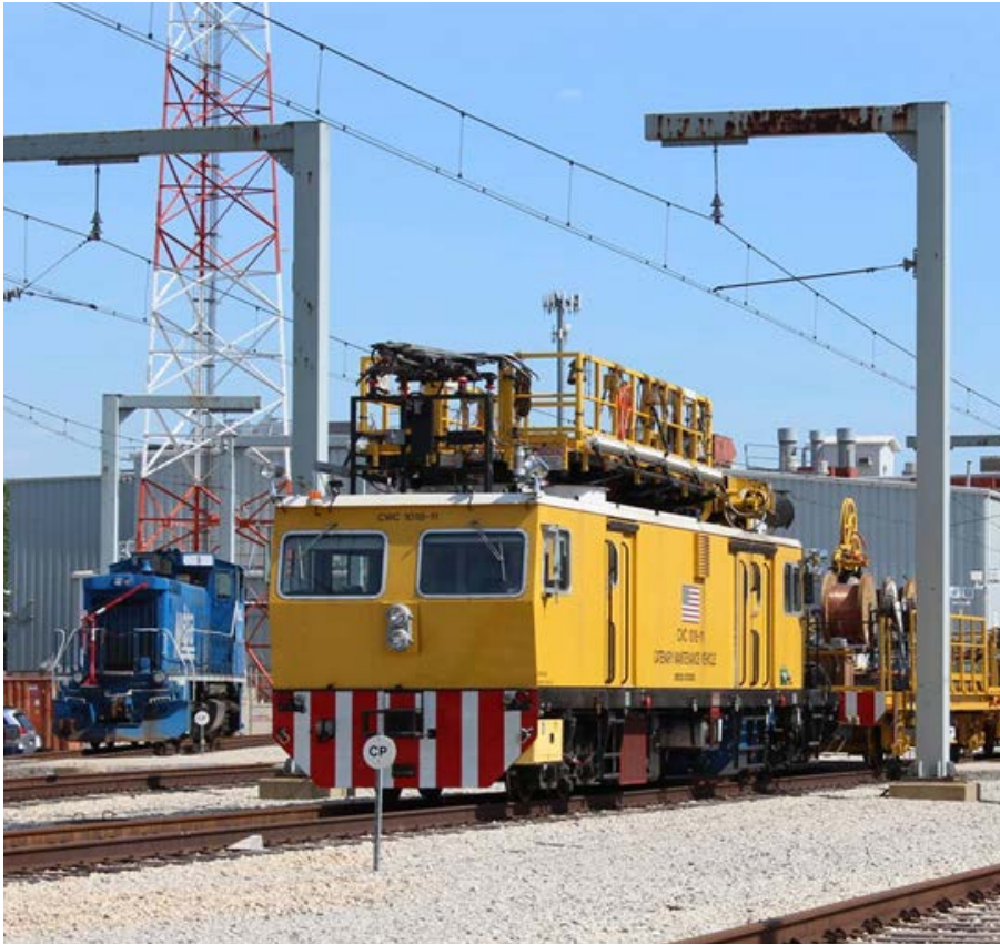
Metra Electric District catenary maintenance vehicle
