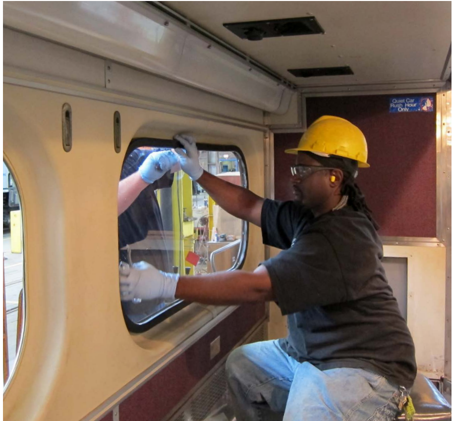
Carman Bryant Howse replaces a window in a car being rehabilitated at Metra's 49th Street Shop
