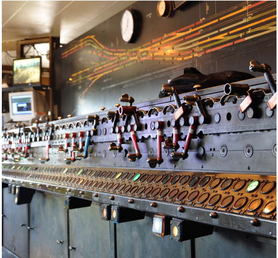
80-year-old manually operated interlocking machine inside tower at A-2 crossing Photo: Mark Llanuza
